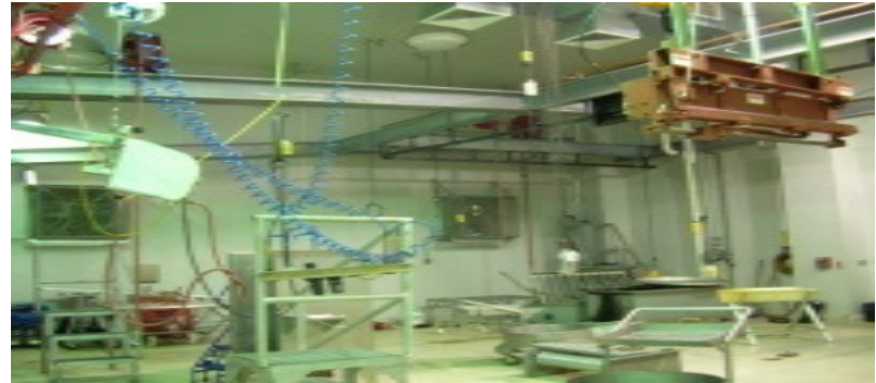
Slaughter and carcass processing facility
